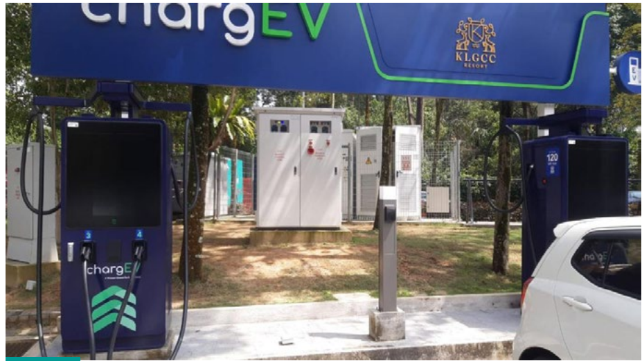
Foto 3: Stesen EVCS yang menyokong mod pembayaran kad kredit/debit Photo 3: EVCS station supporting credit/debit card payment modes
