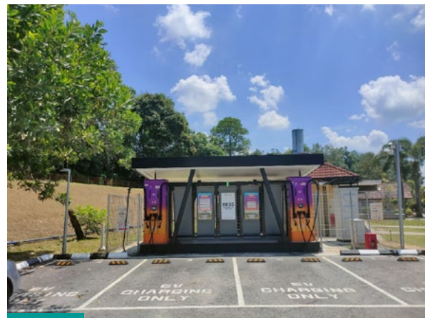
Foto 2: Stesen EVCS di Kawasan Hentian Sebelah Senawang (Arah Utara), Lebuhraya PLUS Photo 2: EVCS Station at Senawang Lay-by Area (Northbound), PLUS Expressway
